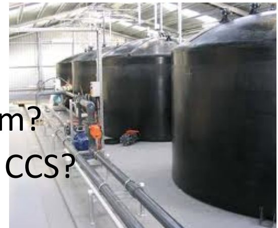
VRB Power Systems flow battery
